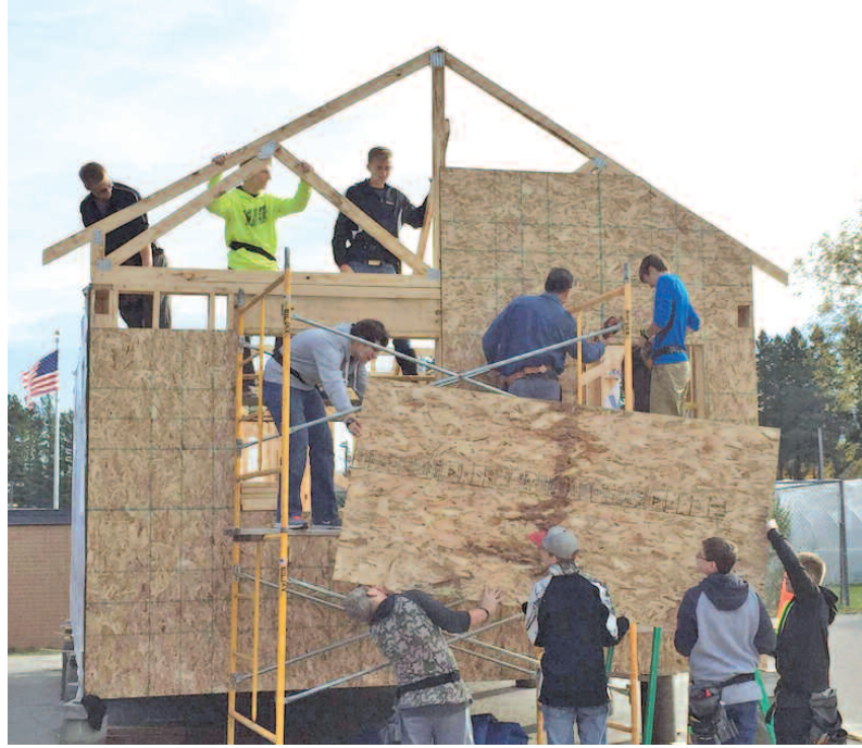
The sounds of hammers pounding have been heard outside of doors of Ellsworth Community School this fall. Those sounds originate from the students of the newly formed Building Trades class at Ellsworth High School. COURTESY PHOTO
